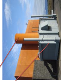
Air intake and exhaust left turbine
