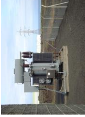
Transformer left turbine
