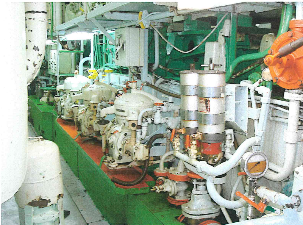
2. Fuel and lubricating oil separators
