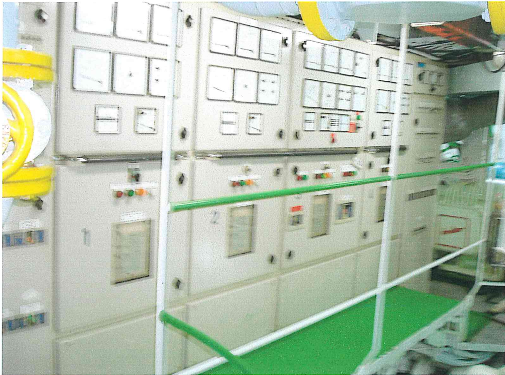
1. Main electrical switchboard in the engine room
