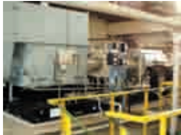
Refrigeration train in an Ammonia plant, Turkmenistan
