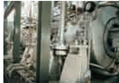
BCL 406/B + BCL 305/C + BCL 305/D compressor driven by MS5002 Gas Turbine installed in Venezuela
