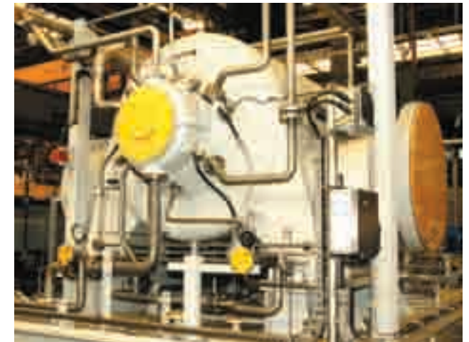
Pipeline Centrifugal Compressor PCL 603
