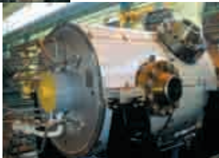
Storage to Pipeline Compressor Gazprom
