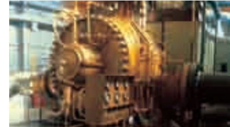
A PCL 1002 booster compressor on the Soyuz gas pipeline
