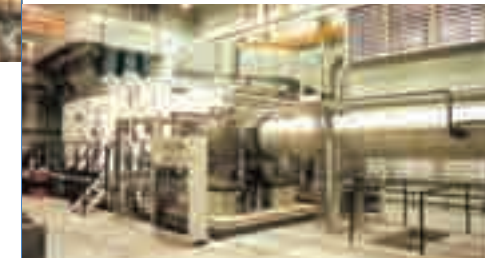
PCL compressor installed in Transcanada pipeline
