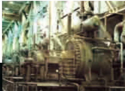
The PCL 802 centrifugal compressor boosting natural gas on board the main Ekofisk platform
