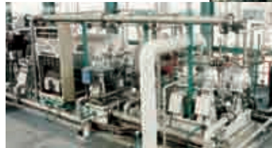
Urea synthesis compressor trains in a petrochemical plant - Qatar
