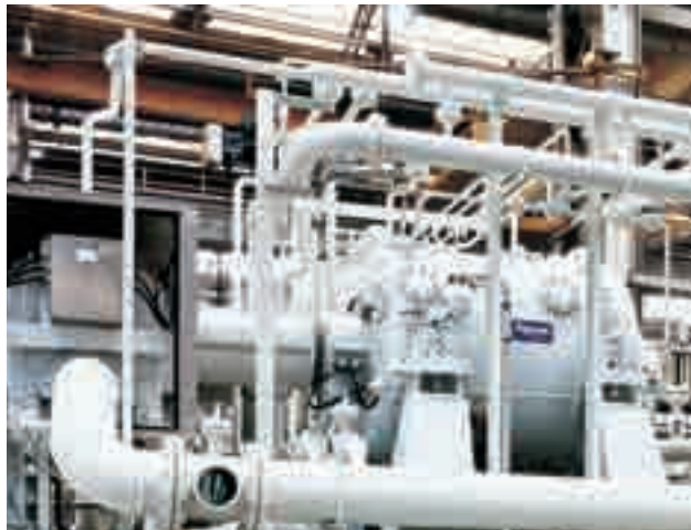
BCL 405/C Re-injection Compressor offshore installation North Sea
