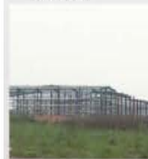
20000m 2 ZAMBIA PLANT
