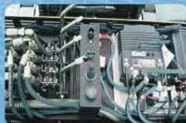
Double controllers with CANbus communication to oil tube and wire
