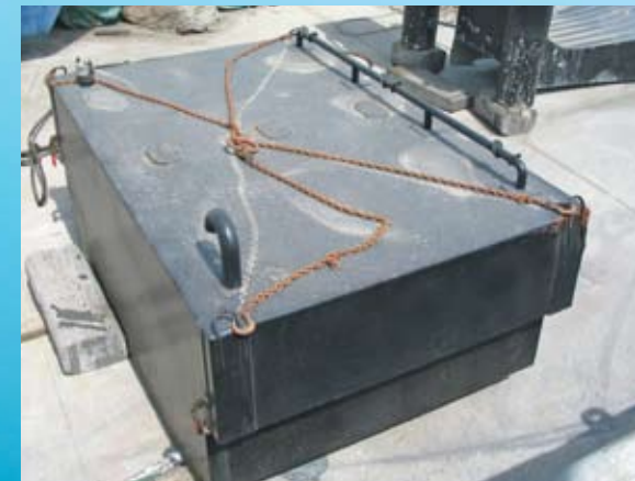
Recuperation oil tank
