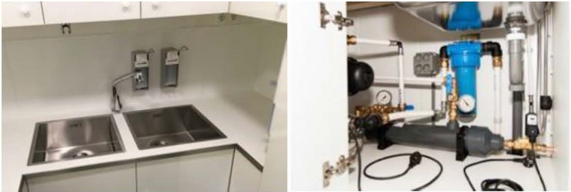
Sinks, cupboards and water treatment system in the middle section of the trailer. The fridge is also located here
