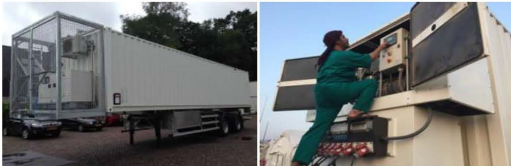
The 20 kVA generator of the surgical trailer (left) and a generator on the storage trailer (right).
