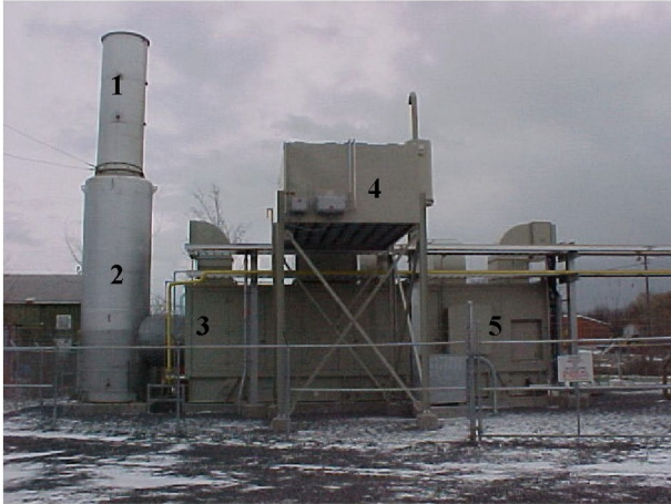
Installed Solar Taurus 70 Gas Combustion Turbine Generator:
