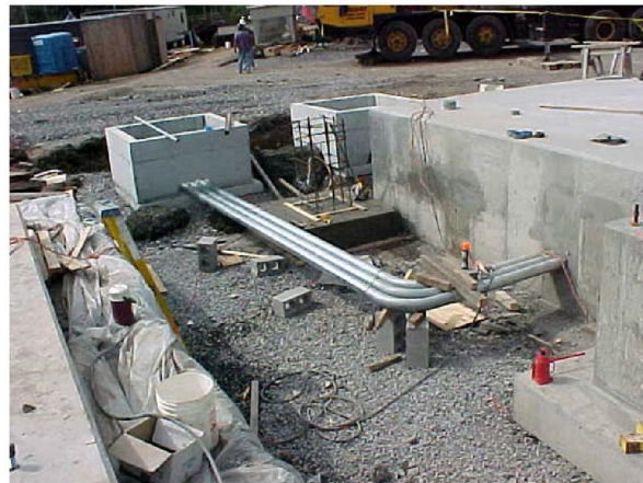
Underground Conduit between Power Control Room Pad (right) and Electric Service Meter Pedestal (upper center); Gas Compressor Pad (left).
