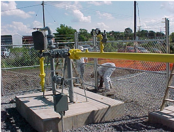
Gas Meter and Gas Line to Gas Compressor.
