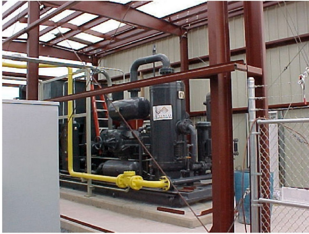
Gas Compressor showing Gas Lines and Skeleton of Enclosure.
