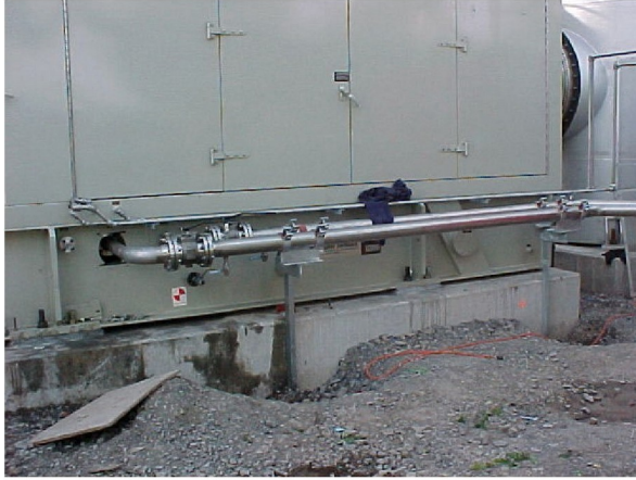
Turbine Wash Down Line to Sump.
