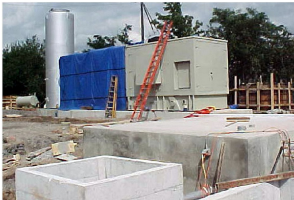
Solar CT with Noise Muffler (background; Pad for Power Control Room (right foreground); Electric Service Meter Pedestal (left foreground).
