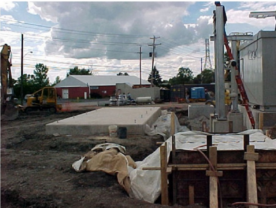
Gas compressor foundation pad (Center); Gas meter pedestal (right foreground); Power Control Room (right).
