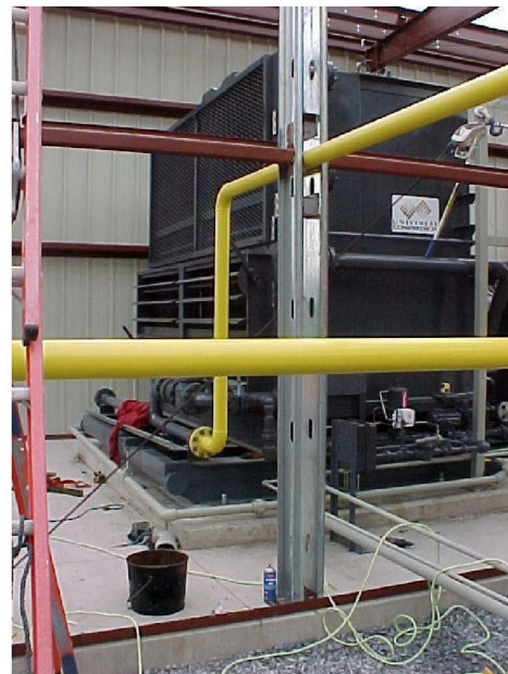
Gas Interconnect with Gas Compressor; Structural Elements of Noise Attenuating Enclosure.
