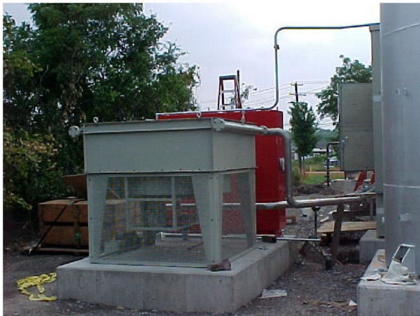
Lube Oil Cooler.
