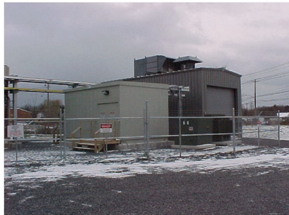
Power Control Room (left center); Gas Compressor Building (right center); Pipe/Cable Trays and CT Generator (Left)
