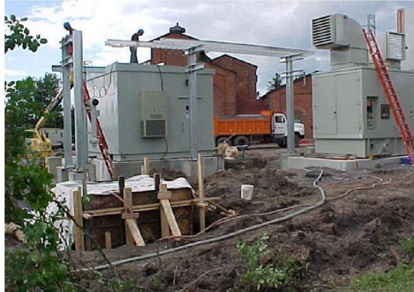
Power Control Room (left); CT Generator (right); Gas Meter Pedestal (foreground).
