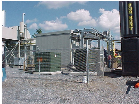
Transformer and Switch Cabinet (foreground); Power Control Room (behind); Solar CT and Air Intake Structure (background).
