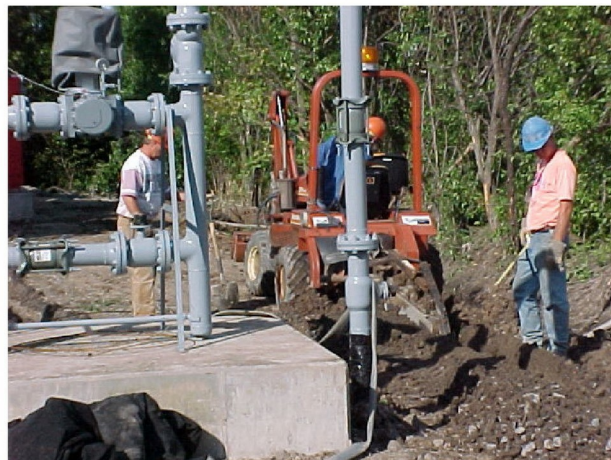
Gas Meter Interconnect.
