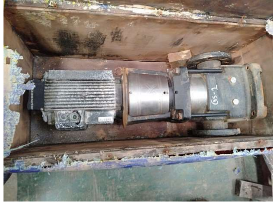
LT circuit circulation pump
