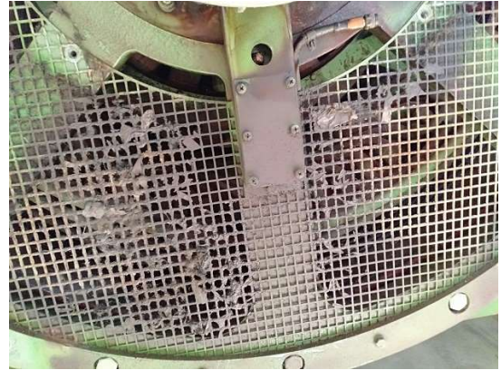
Main winding (BOTTOM)
