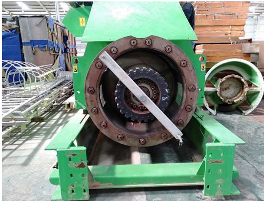
Generator rotor lock bar
