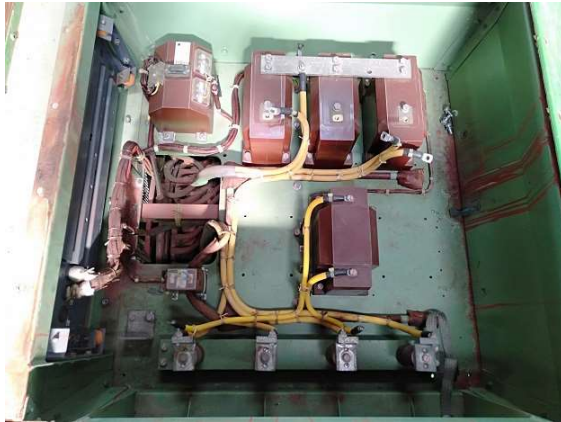
Main terminal box
