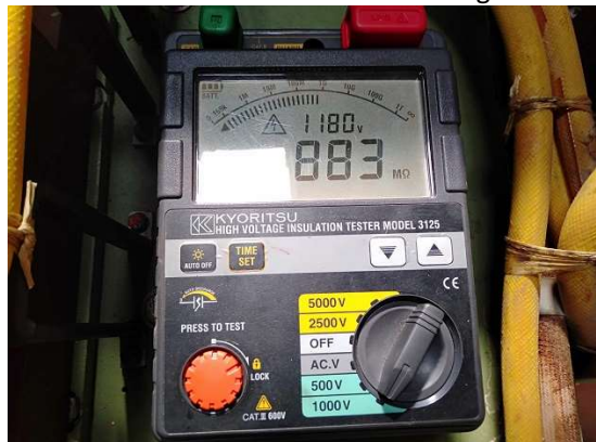
Phase W insulation resistance: 883 mega ohm
