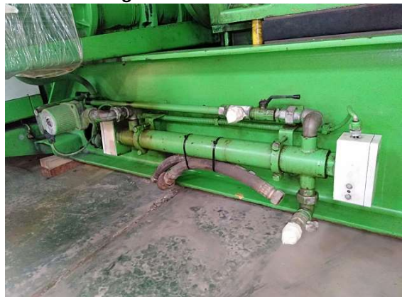
Pre-heat cooling water
