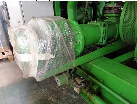
Jacket water pump
