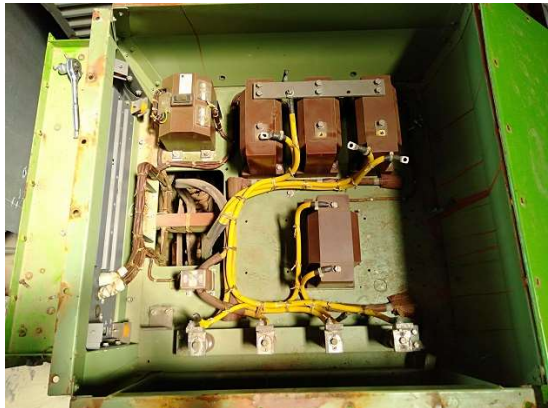
Main terminal box
