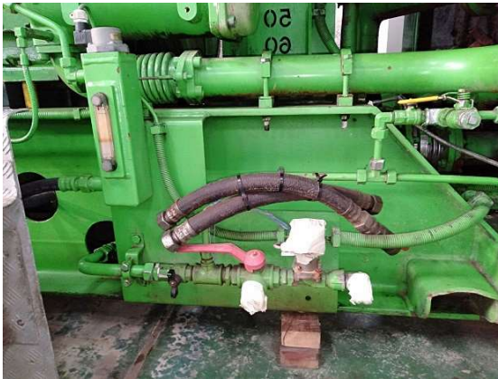
Oil inlet & discharge lines and oil level
