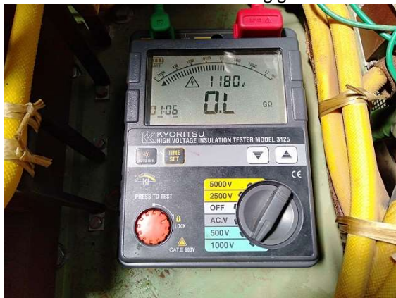
Phase V insulation resistance: >1 giga ohm
