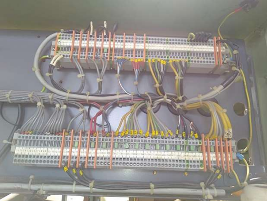
Exciter/AVR interfacing terminals
