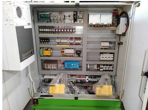
Interface panel inside view
