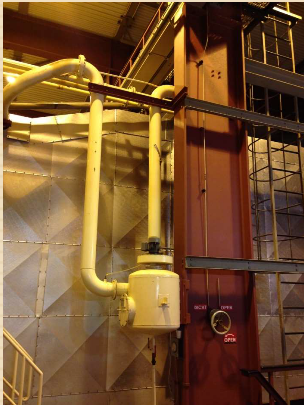
Inside power plant
