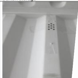
Sealed air hole
