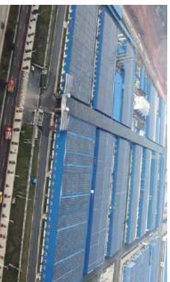
麓谷科技园12.82MW金太阳工程 LUGU Science Park 12.82MW PV power plant(Golden sun project)
