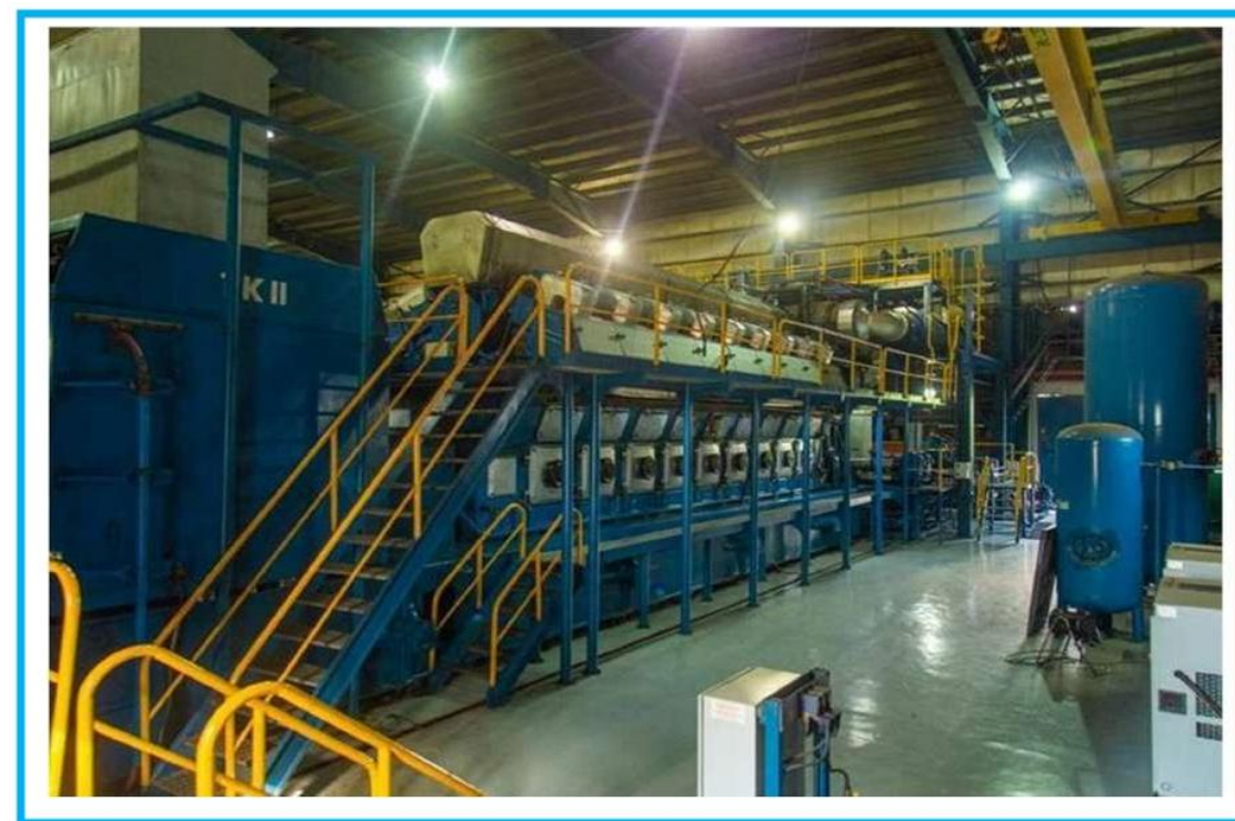
ENGINE ROOM BOTTOM FLOOR (ENGINE STARTING AIR COMPRESSOR AND AIR RECEIVER)
