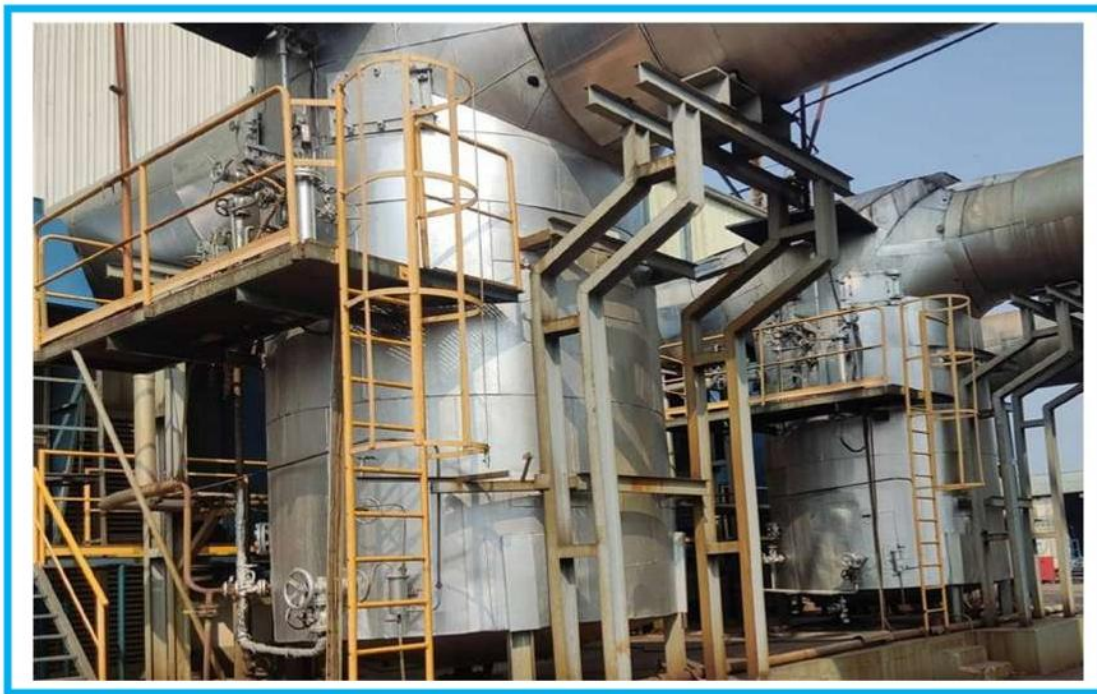
EXHAUST GAS BOILER
