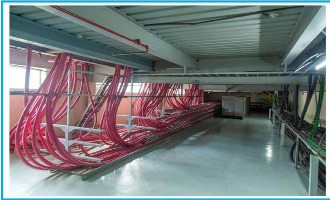
HIGH VOLTAGE CABLE ROOM
