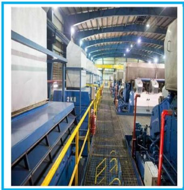
ENGINE ROOM TOP FLOOR
