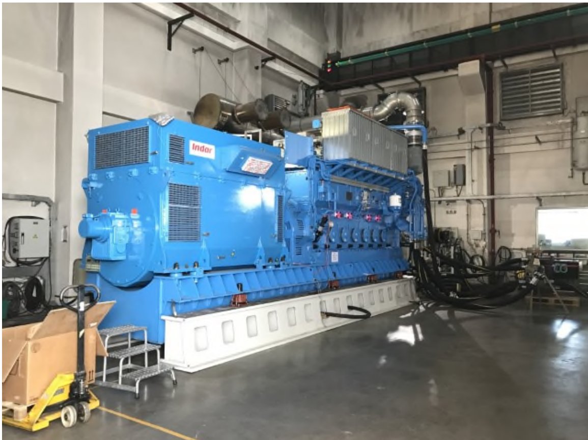
Fig 3: B33:45 L6 Genset on test bench
