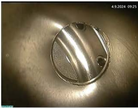
Burner #10 Premix gas passage
