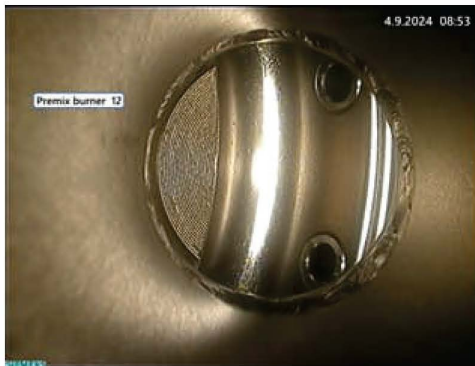
Burner #12 Premix gas passage
