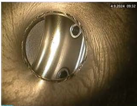
Burner #14 Premix gas passage
