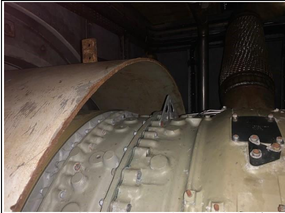
Picture 01: Magnesium casing (12 o'clock)
