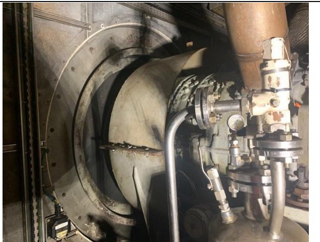
Picture 04: Inlet compressor side (LHS)
