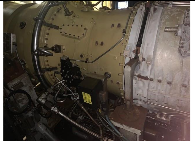
Picture 02: GT RHS
