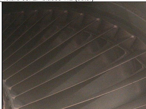
Picture 05: LP blades overview
