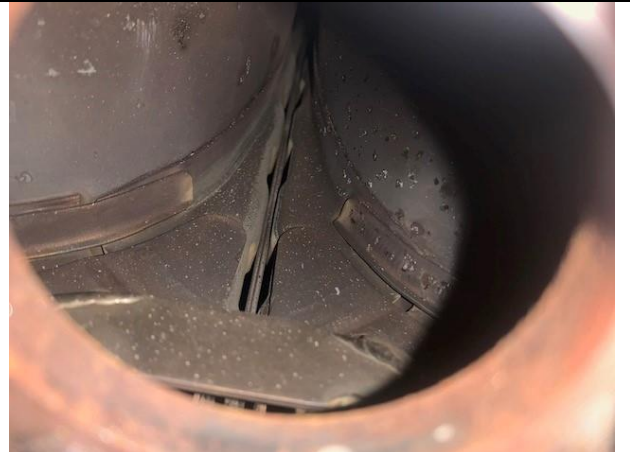
Picture 12: combustor outer liners
