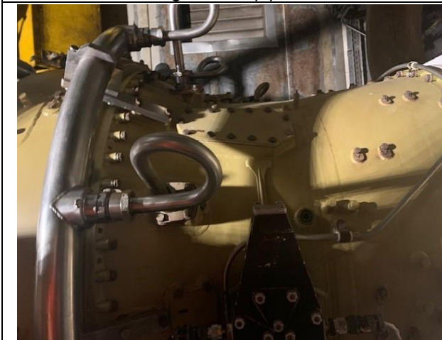
Picture 03: Fuel manifold
