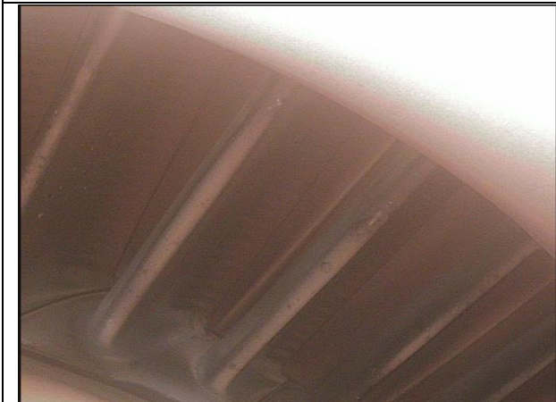
Picture 05: HP turbine nozzle & L.E Blades #7
