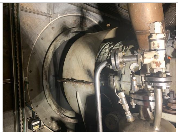
Picture 02: IGV rods and arms (RHS)
