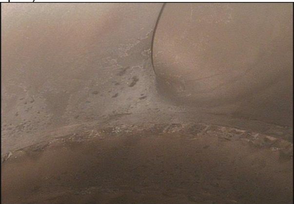
Picture 09: combustion chamber #7 (minor burn spots)
