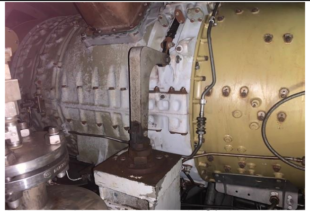
Picture 02: Magnesium casing LHS (minor corrosion)
