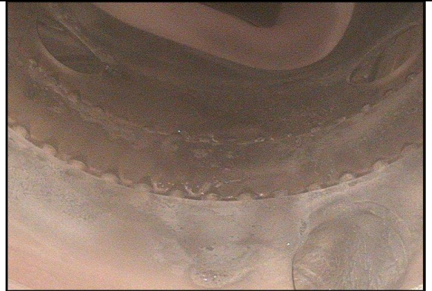
Picture 06: combustor #3 combustion chamber (minor burn spots)
