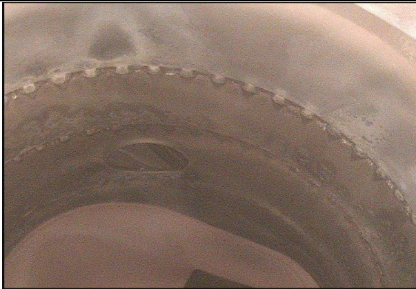
Picture 05: combustion chamber #3 (minor burn spots)
