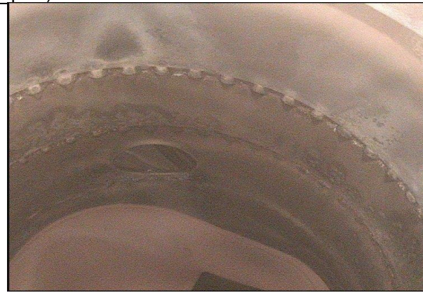
Picture 07: combustion chamber #3 (minor burn spots)
