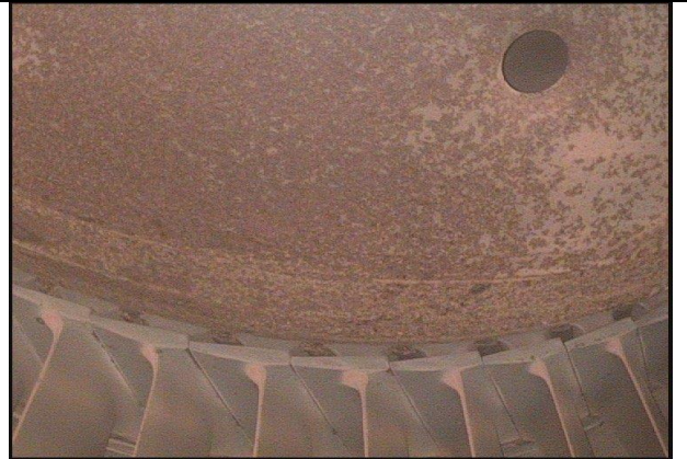
Picture 08: LP blades root & inner cone (minor corrosion)
