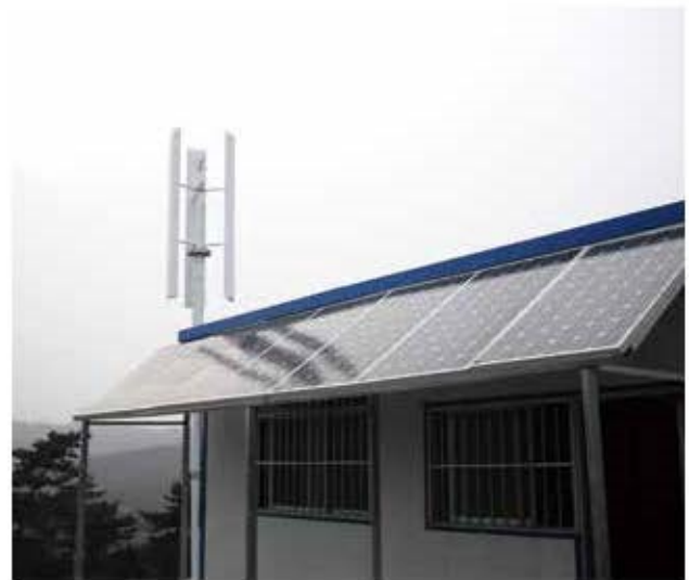
Wind & solar hybrid power supply system installed in Mountain Landscape
