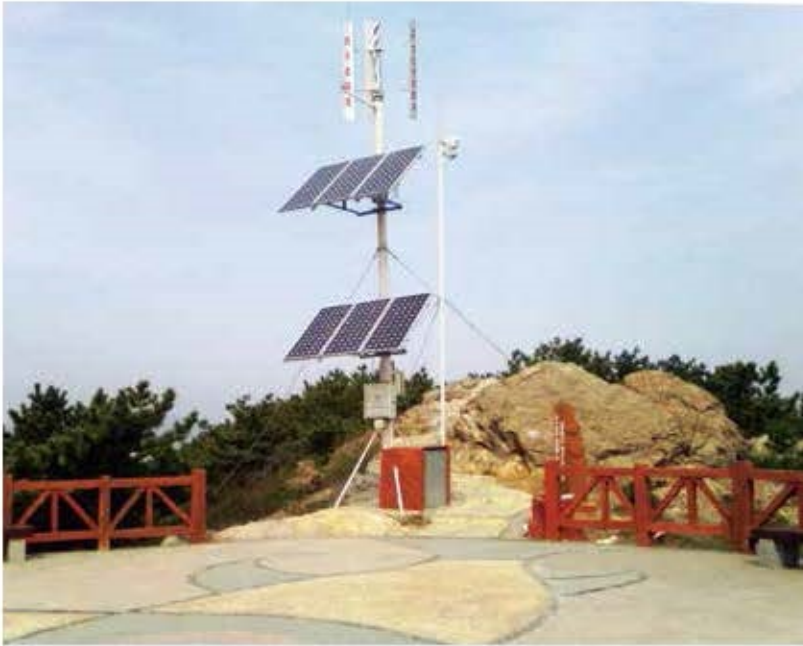
Wind & solar hybrid power supply system for monitoring installed in viewing tower in Dalian City
