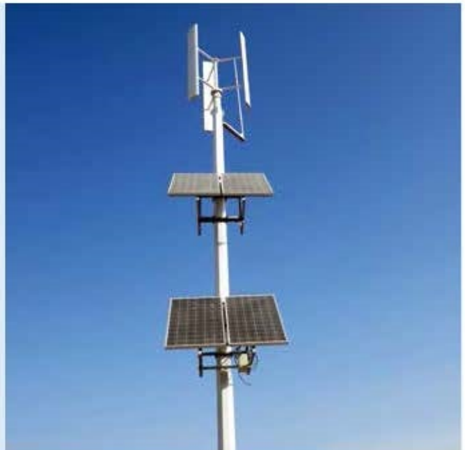
Wind and solar power system for monitoring in Sinkiang
