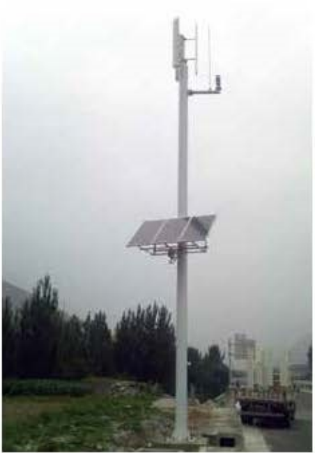
Wind & solar hybrid power supply monitoring system installed on Expressway in LongNan City
