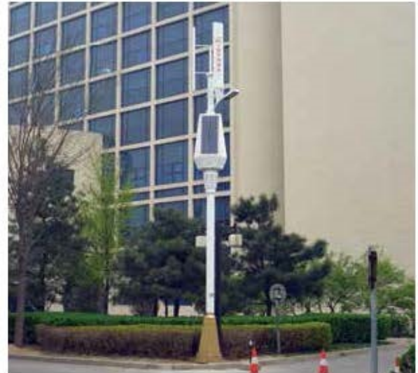
Wind & solar hybrid power supply lighting system installed in Zhongguancun in Beijing
