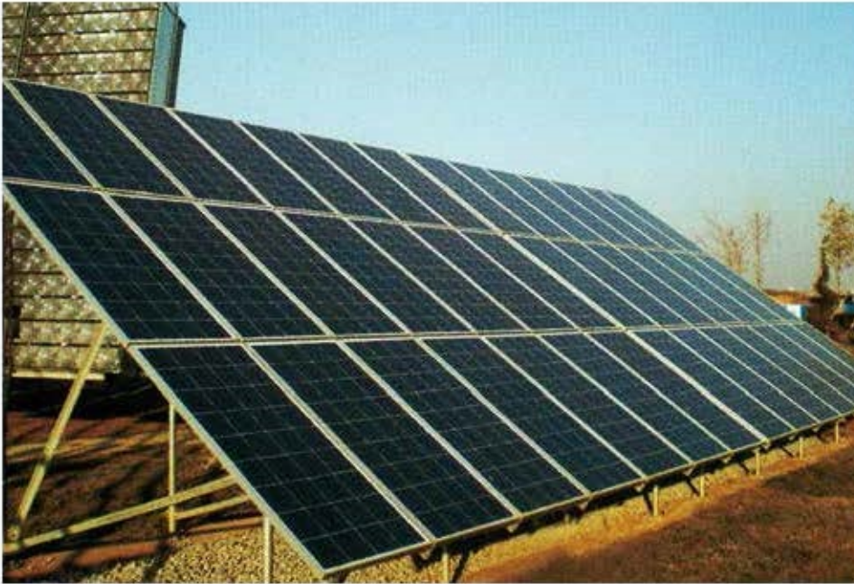
Solar power supply system installed in Langfang City, Hebei Province
