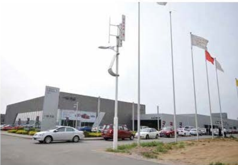
Wind & solar hybrid power supply lighting system installed in Tangshan automobile town
