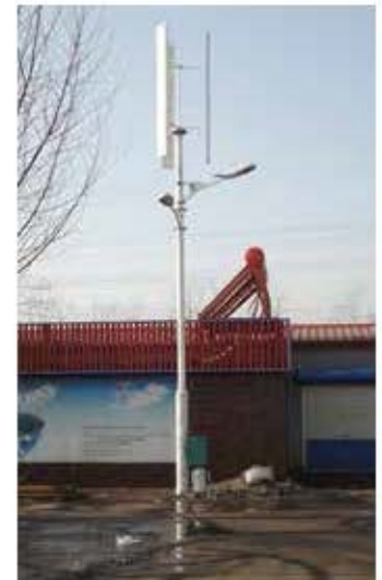
Wind power supply system used in house
