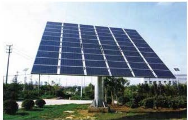
Small micro-grid power supply system at expressway exit
