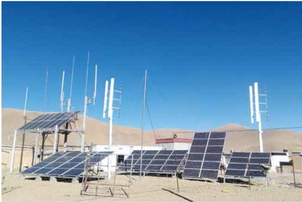
Wind solar hybrid system equipment in Xinjiang
