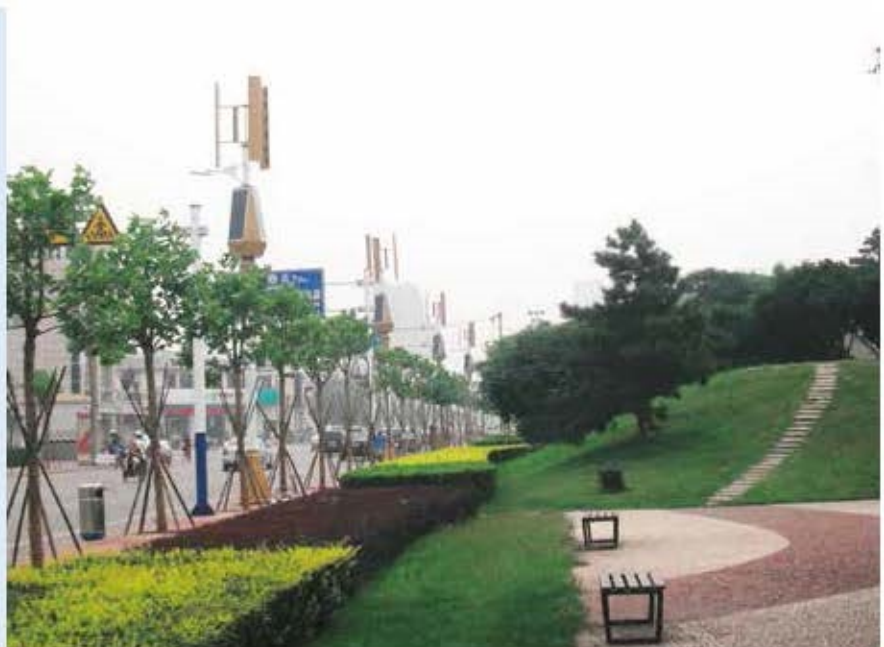
Wind & solar hybrid power supply lighting system in park
