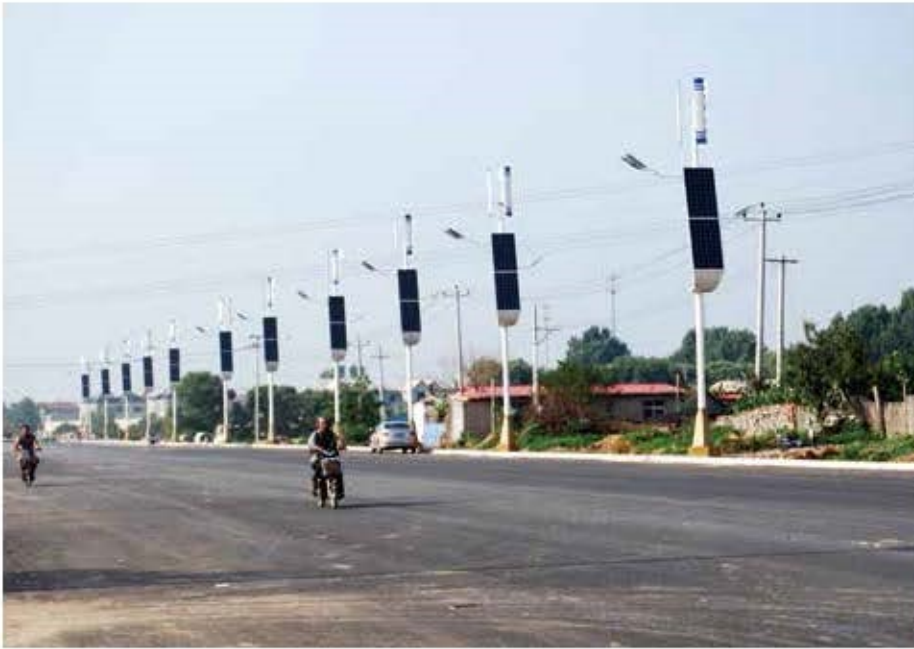
Wind & solar hybrid power supply lighting system in State Road
