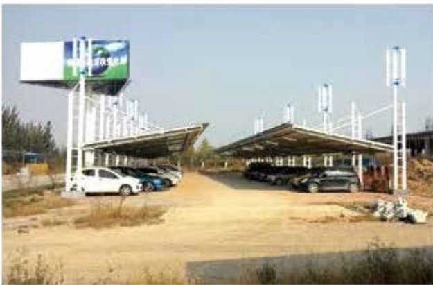
Wind & solar hybrid power supply equipment
