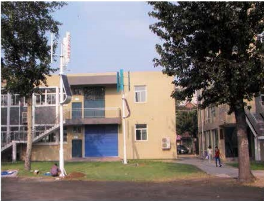
Wind & solar hybrid power supply lighting system installed in campus.
