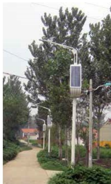
Solar street light installed in Yutian Town
