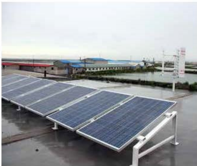
Wind & solar hybrid power supply system installed in Mariculture base
