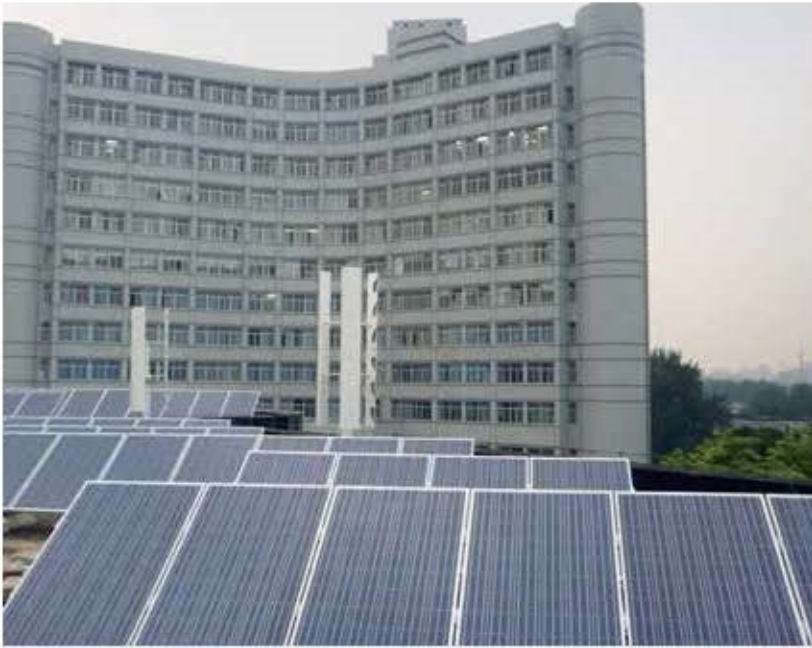
Wind & solar hybrid power supply system Installed on roof in Beijing
