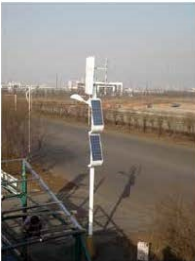
Wind & Solar hybrid power supply lighting system on Shangjin Road, Haigang
