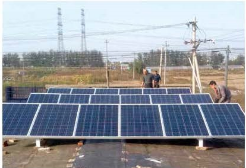
Small micro-grid power supply system in Beijing Logistics Park
