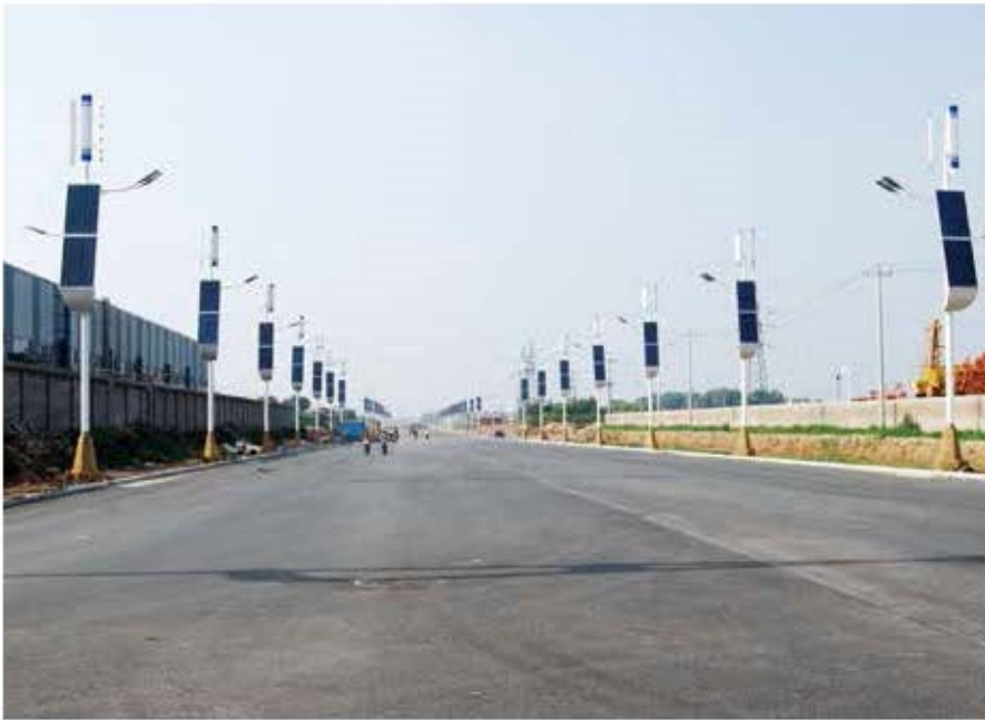
Wind & solar hybrid power supply lighting system installed at the sides of expressway in the 6-lane
