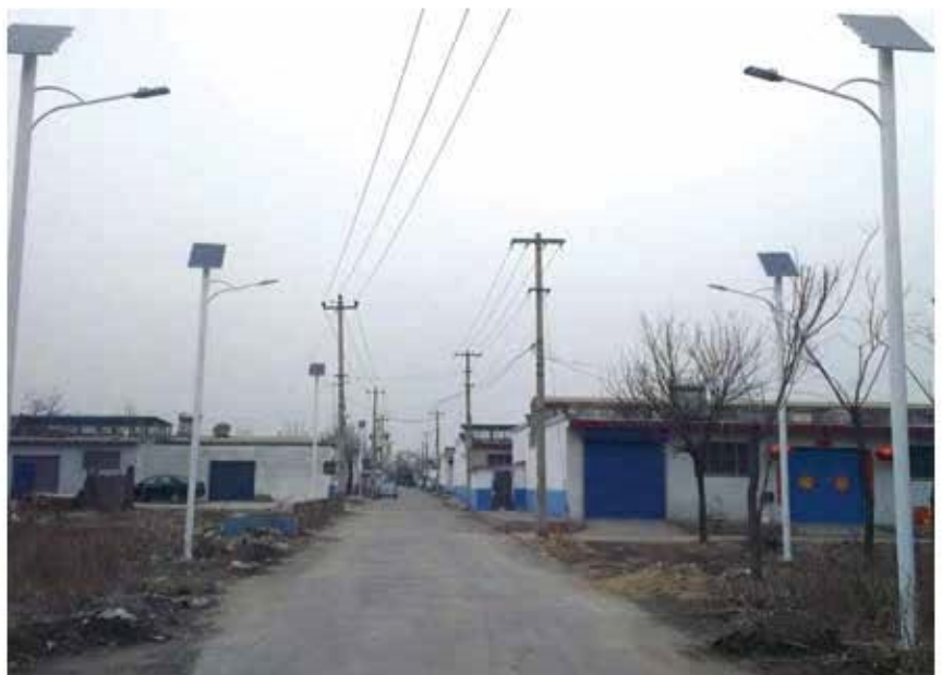
solar street lamp at village of Lubei
