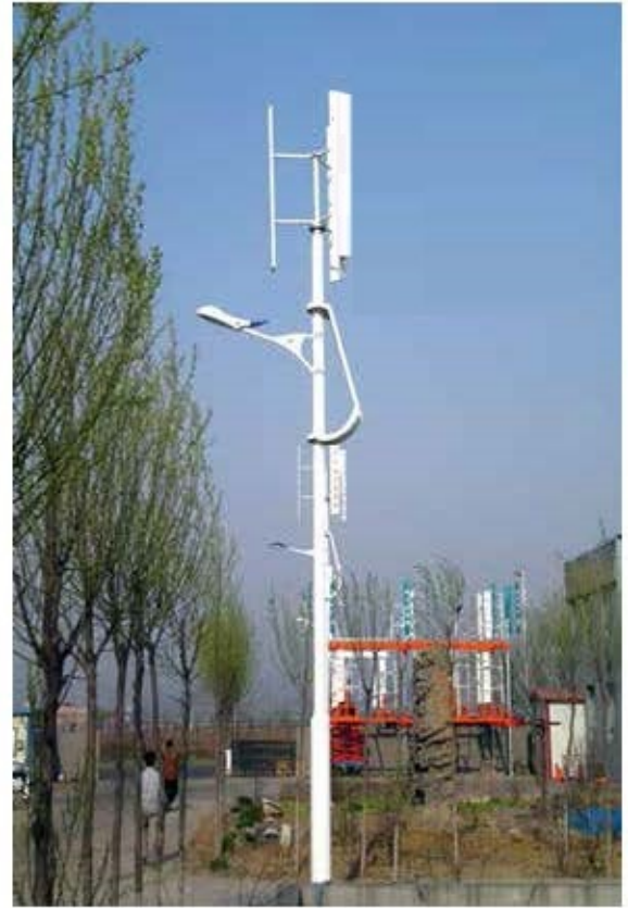
Wind & solar hybrid power supply lighting system in Haigang Factory
