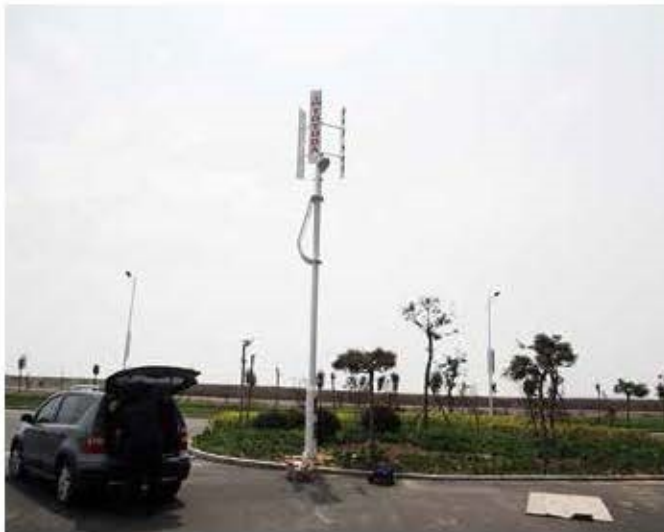
Wind & solar hybrid power supply lighting installed in Shougang Group wharf
