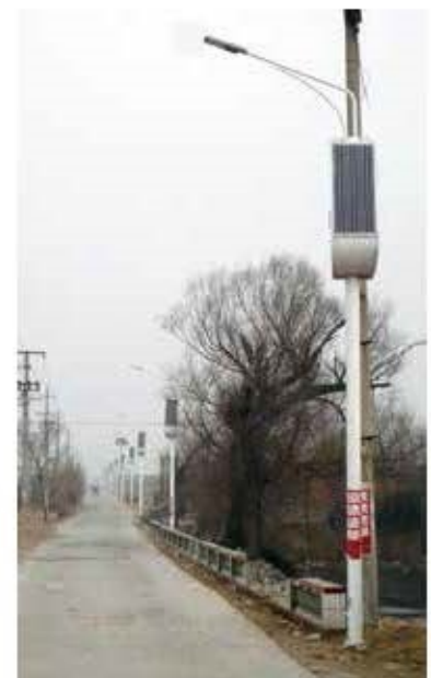
Solar street lamp intalled at Town Laoting
