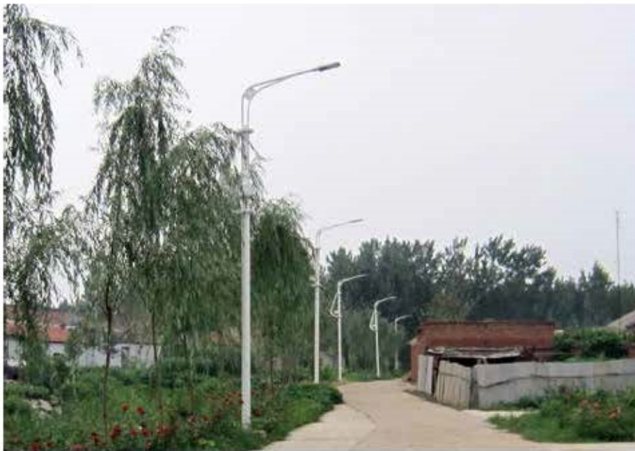
Solar lighting system installed in suburb
