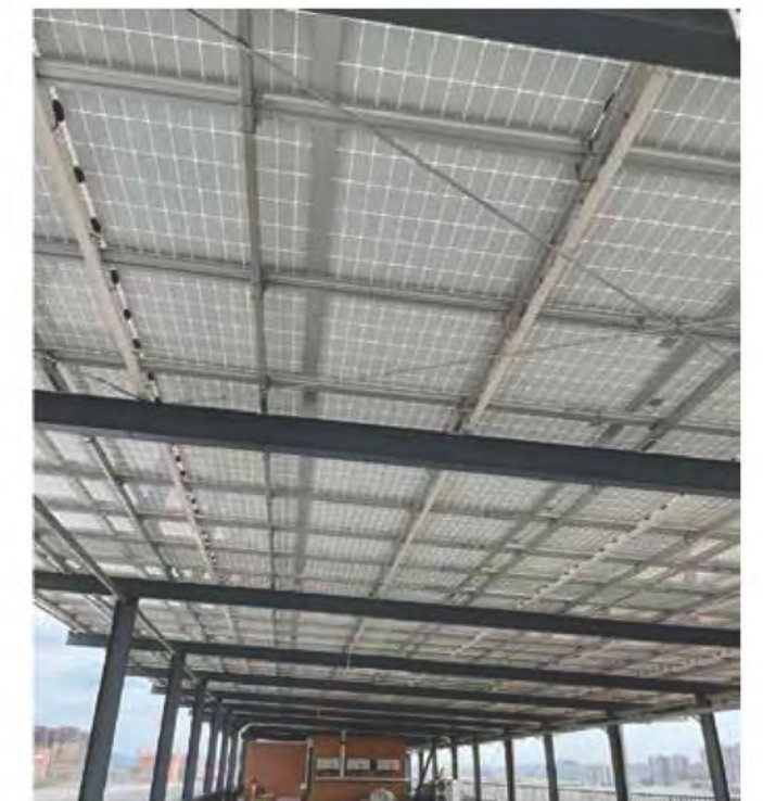
DONGGUAN 1MW PHOTOVOLTAIC PROJECT
