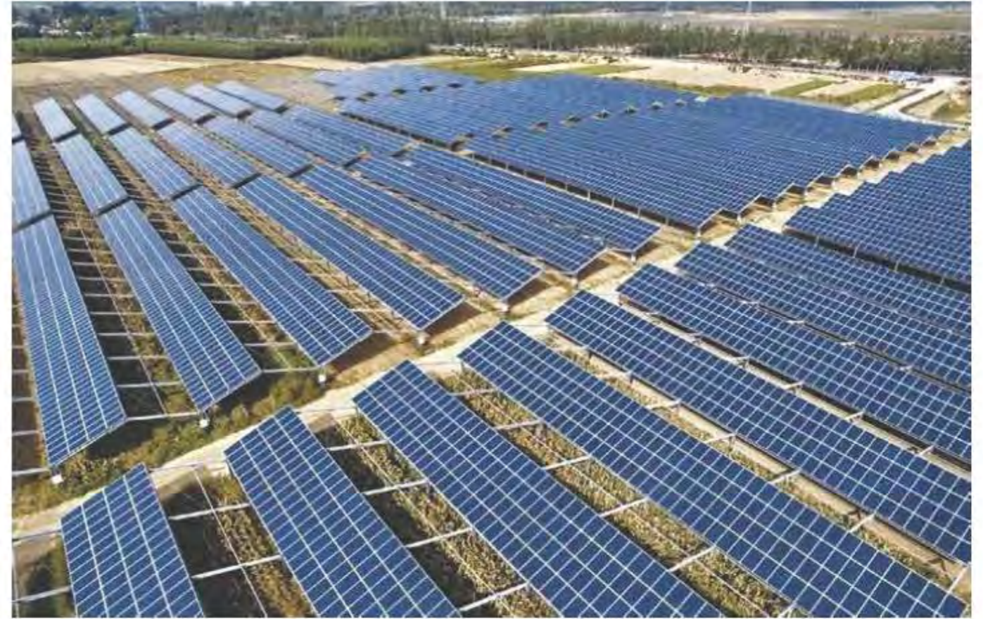
HEBEI 1.2MW POVERTY RELIEF GROUND PHOTOVOLTAIC POWER STATION
