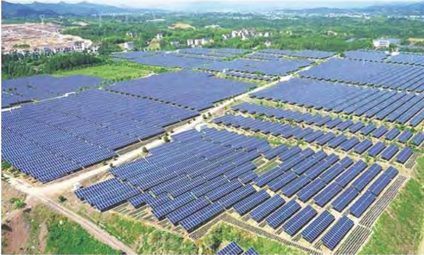
SHAANXI 6.28MW POVERTY RELIEF GROUND PHOTOVOLTAIC POWER STATION
