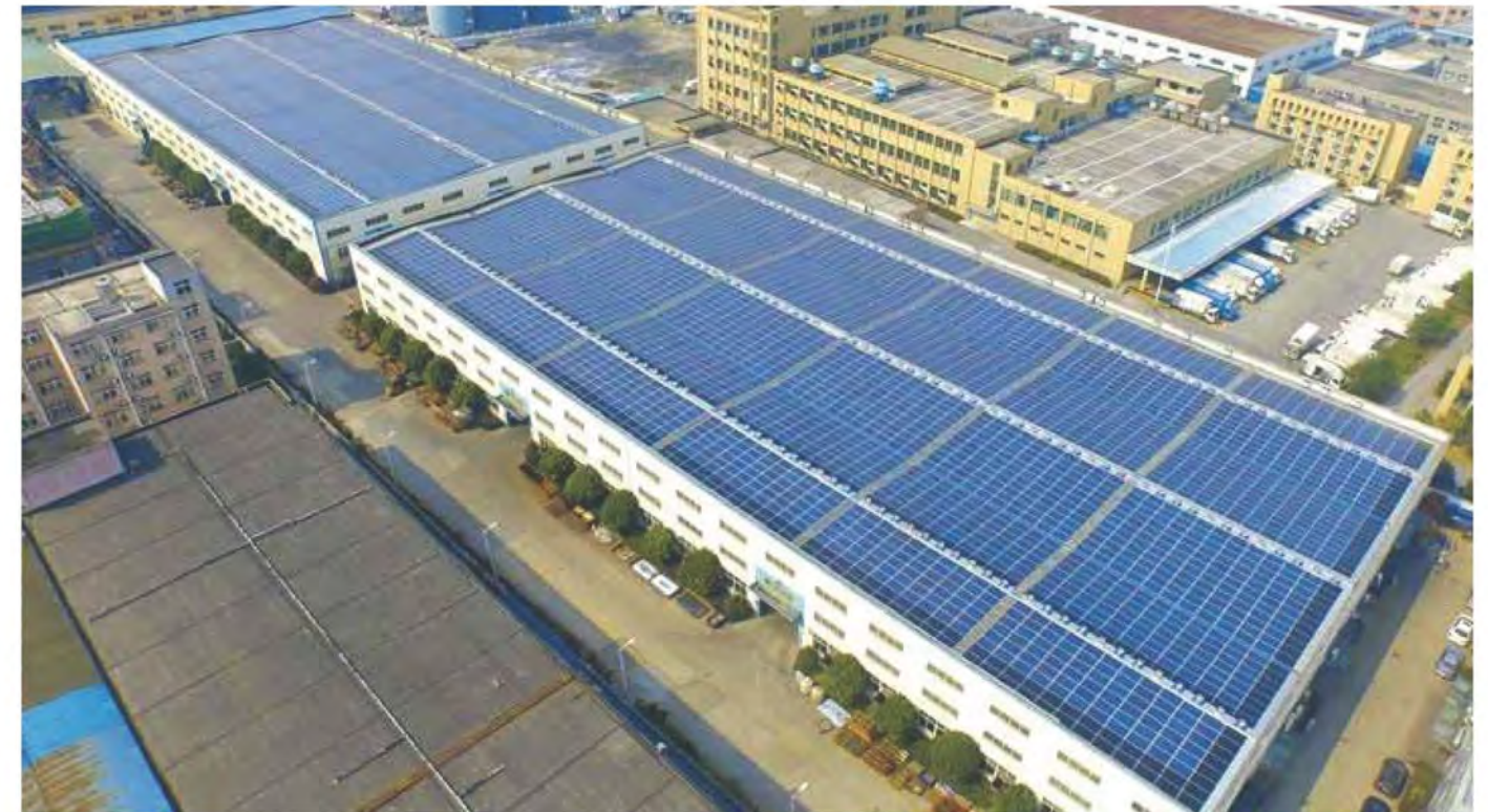
XINJIANG 2MW ROOFTOP PHOTOVOLTAIC POWER STATION
