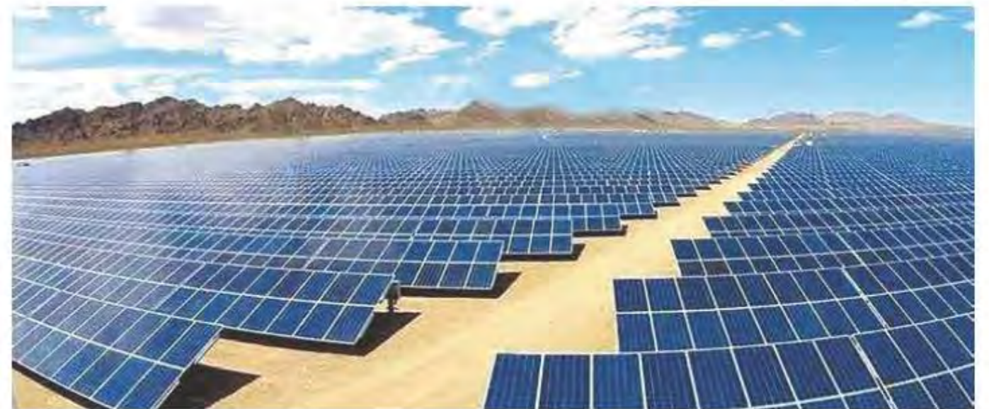
SHANXI 1.2MW POVERTY RELIEF GROUND PHOTOVOLTAIC POWER STATION
