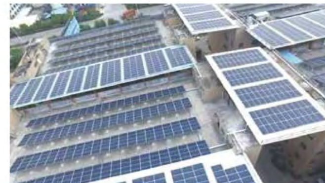
DONGGUAN 1MW PHOTOVOLTAIC PROJECT
