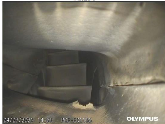
HP Vane coating blistered and spalled.
