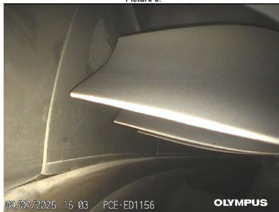
Light rubbing marks on LP Shrouds.
