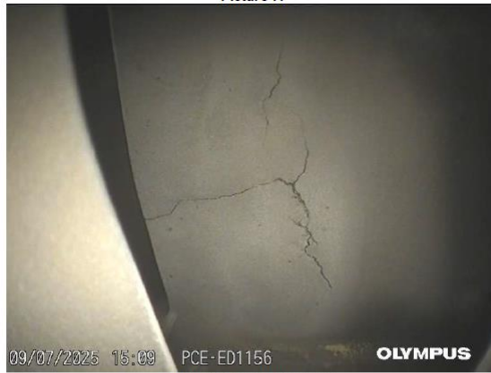
LP Vane converging cracks.
