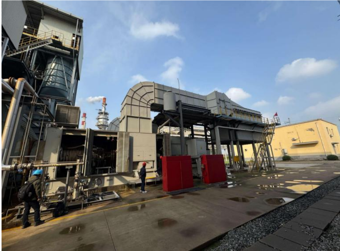
Overall photo of the gas turbine
