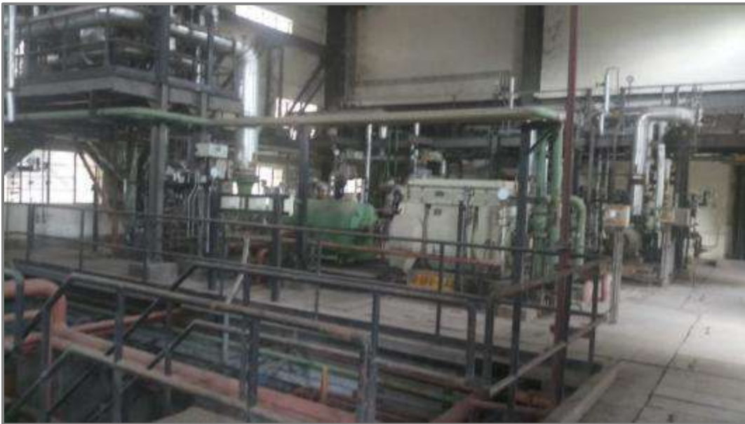
Steam Turbine Auxiliaries
