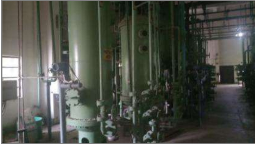
DM Water Plant
