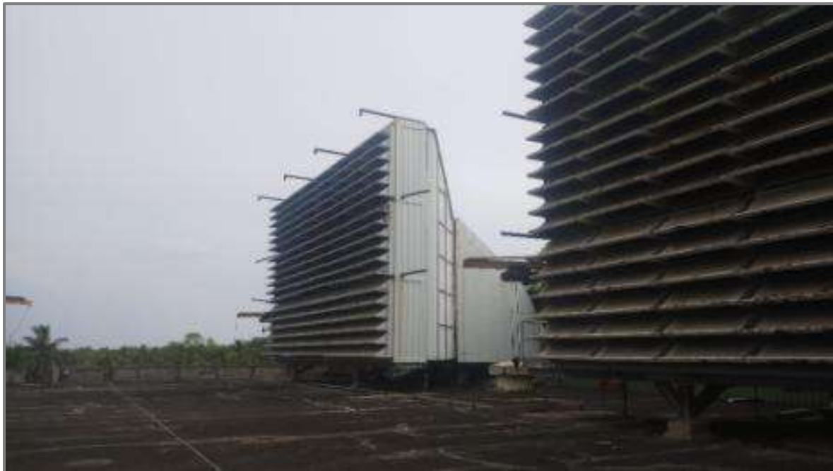
Inlet Filter House of GT # 1A and 1B
