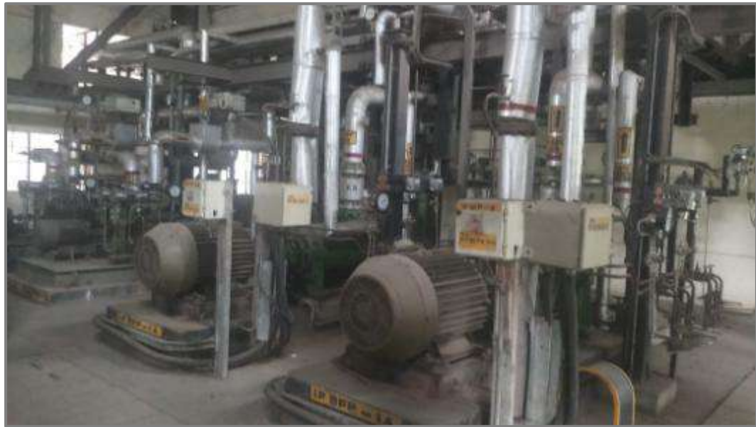
Condition of IP Boiler Feed Pumps
