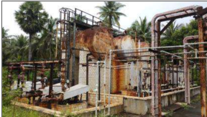
Tanks for DM plant
