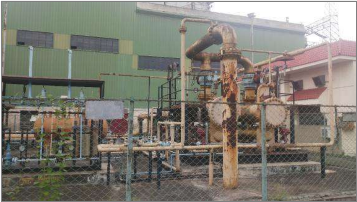
Gas Conditioning Skid
