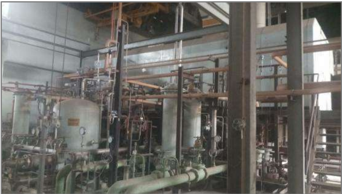
Gas Turbine Generator & Auxiliaries
