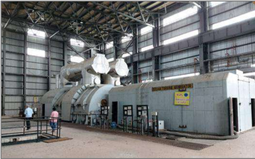
Steam Turbine & Generator
