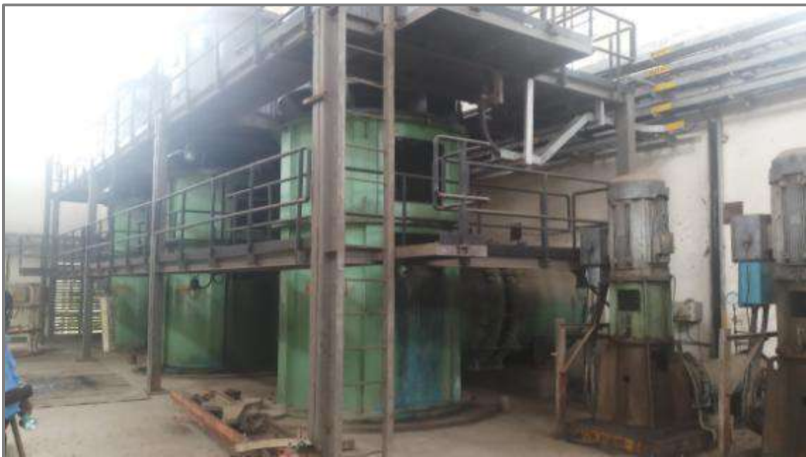
Cooling Water Pumps
